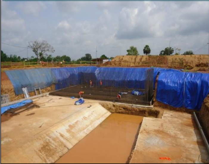
Clear Water Tank, Sasthrikulam
