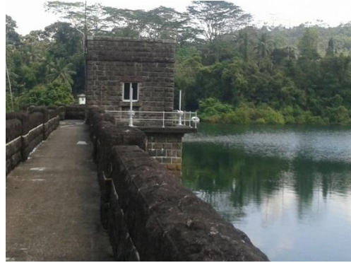
Kalatuwawa Reservoir & Intake Well
