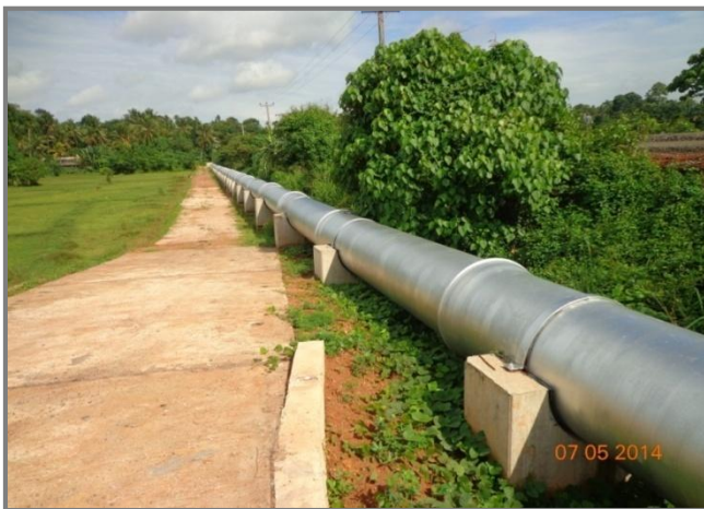
Exposed pipes at Gammanpila tank bund (Kesbewa-Bandaragama Road)
