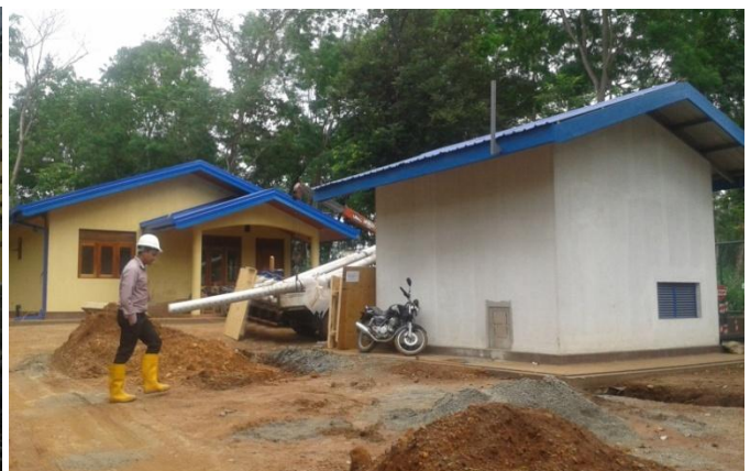
Maduwanwela booster pump house
