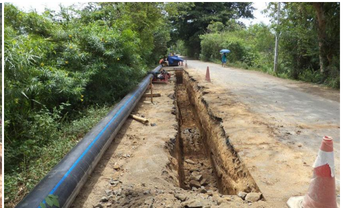
Treated water transmission main
