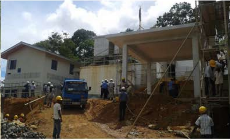
Water treatment Plant
