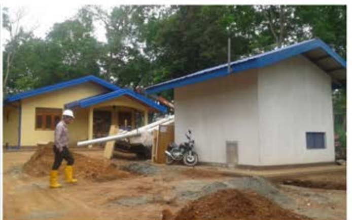
Maduwanwela booster pump house
