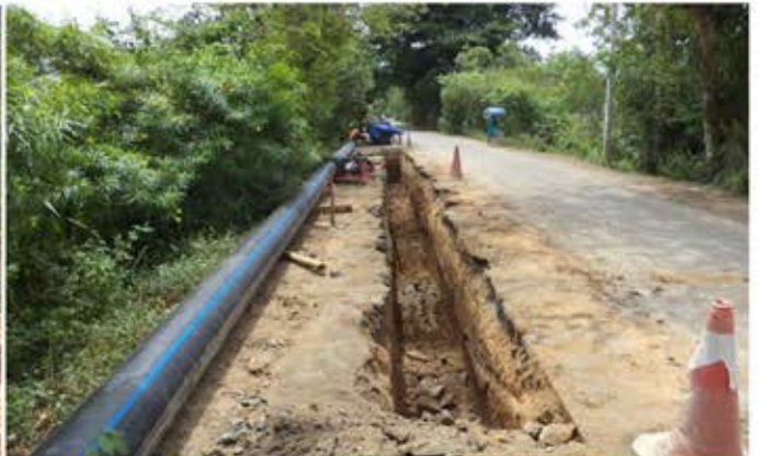
Treated water transmission main
