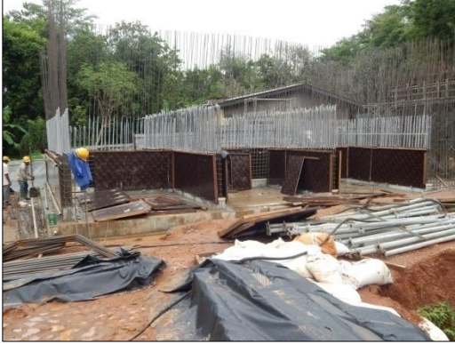
Rapid Sand Filter
