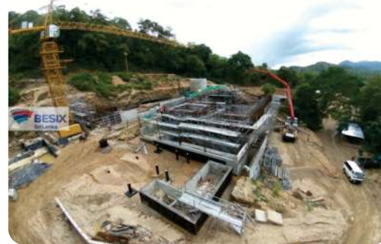
Kumbukkana treatment plant
