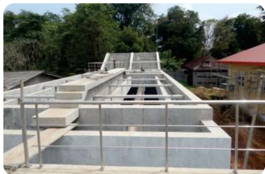
Water Treatment Plant in Mahiyanganaya
