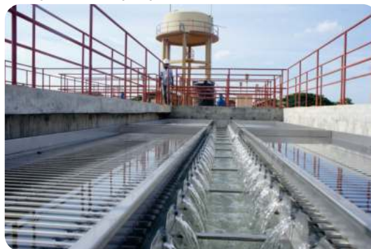
Plate Settlers of Muttur Water Treatment Plant
