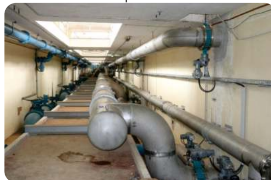
Back wash pumps at Kalatuwawa
