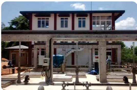
Intake and Raw Water Main of Greater Dambulla WSS
