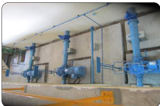
Kandana Pump House
