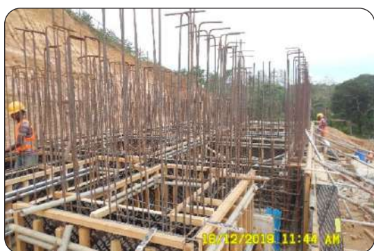
Coagulation & flocculation tanks
