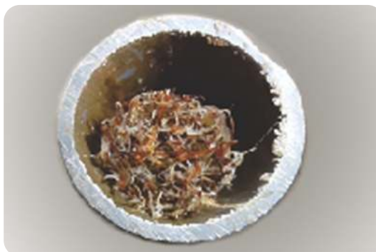
Effects of an undetected leak - roots grown inside a pipe
