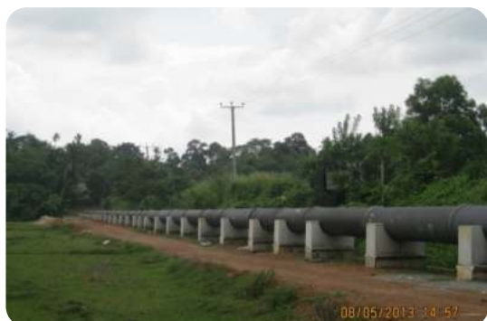
Exposed pipes at Gammanpila tank bund (Kesbewa - Bandaragama Road)
