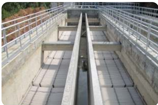
Minneriya /Hingurakgoda Water Supply Scheme
