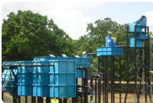
Kilinochchi Water Supply Scheme
