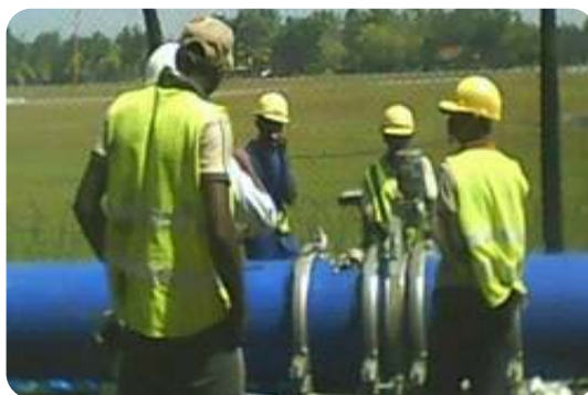
Supply and Laying of 4.5 km, 600 mm diameter DI/PE Pipe line from Maggona to Beruwala
