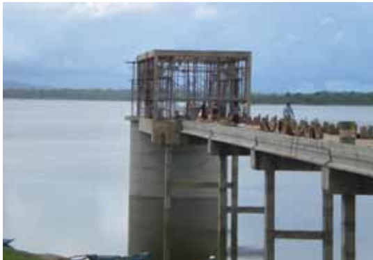
Batticaloa Intake Structure
