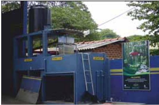
Wastewater Treatment Plant in a Service Station
