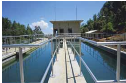
Ragala Water Treatment Plant
