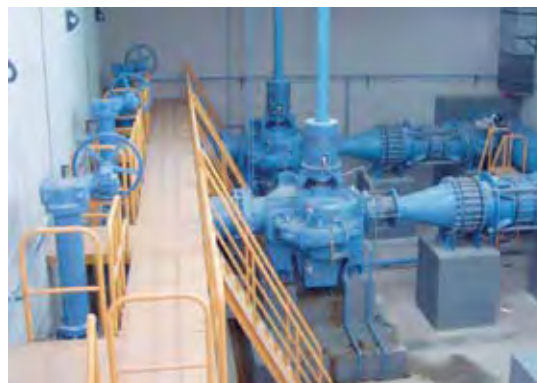
Ambatale Pump House
