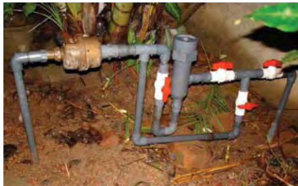
Air Release Valve
