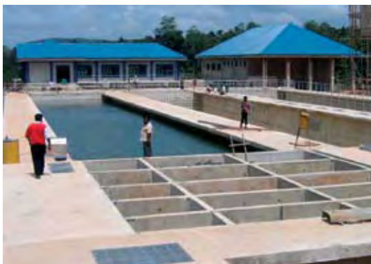
Flocculation and Sedimentation Tanks
